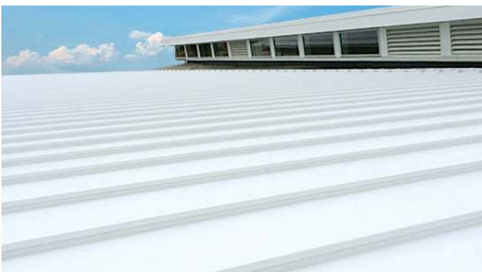
Pictured Above Project: Homes Jr. High School Architect: Robin Randall with Legat Architects Installing Contractor: Metalmasters Color: Shasta White
